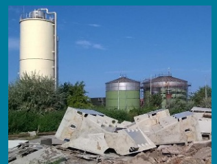
Old EGSB internals replaced by Paques
