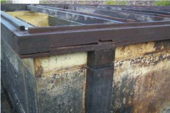
1. Damaged wooden frames.
